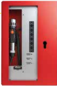
Digital fire brigade call station FWDSP-PZ
